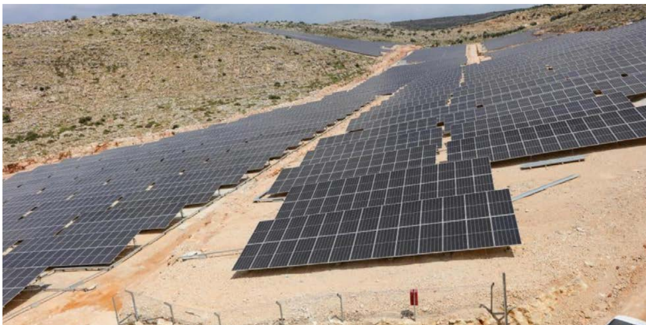
Figure 38: Solar Power Plant in Deir Abu Mashal
